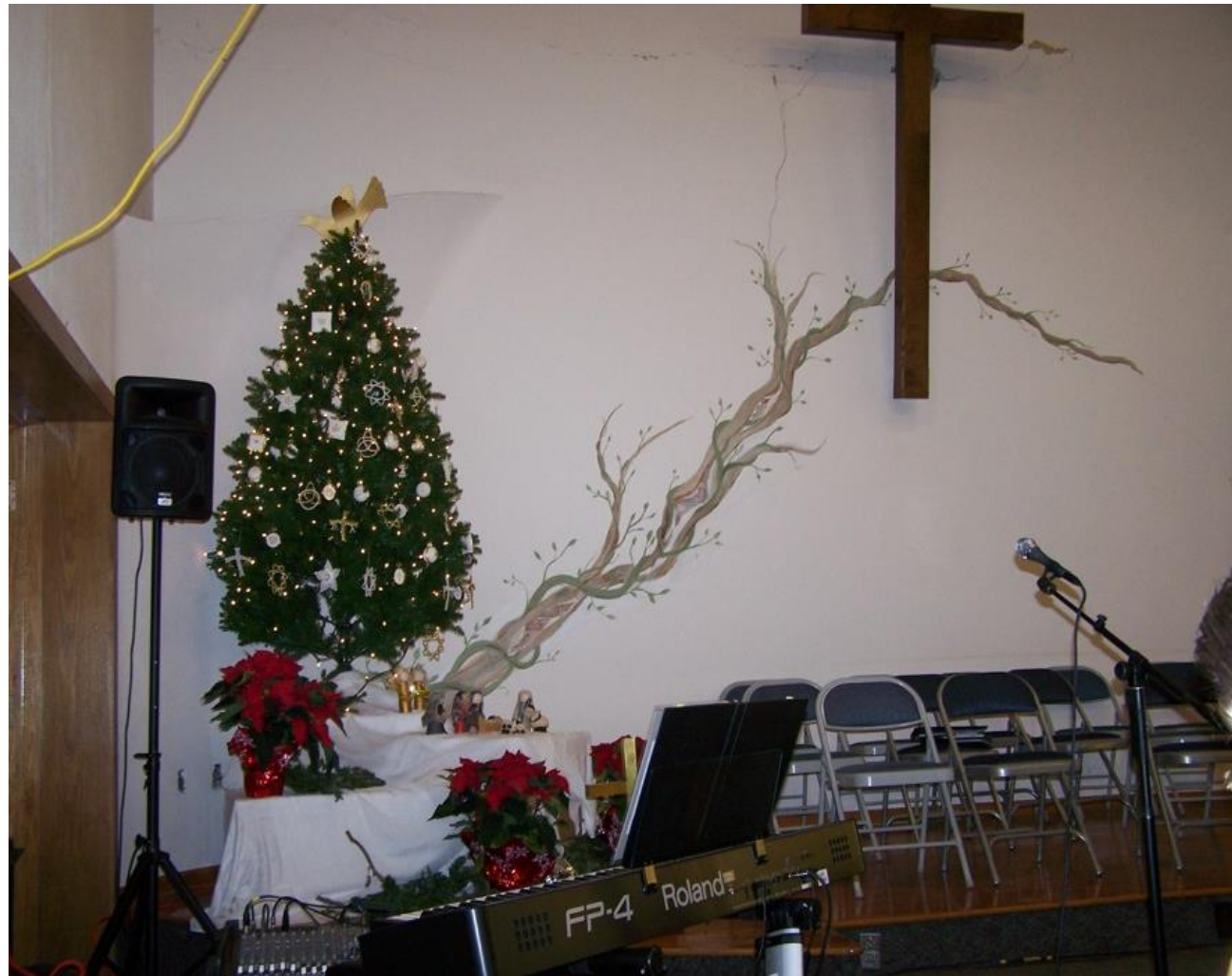
East wall of sanctuary at Christmas. Sharon Jones' whimsical art work covers crack in plaster.
