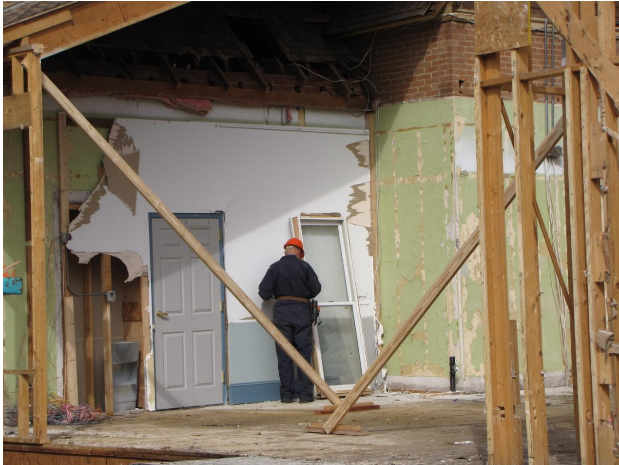
A part of Centennial Room (looking NW). Note masonry wall of original sanctuary in top right. Entrance to south hallway at bottom center.
