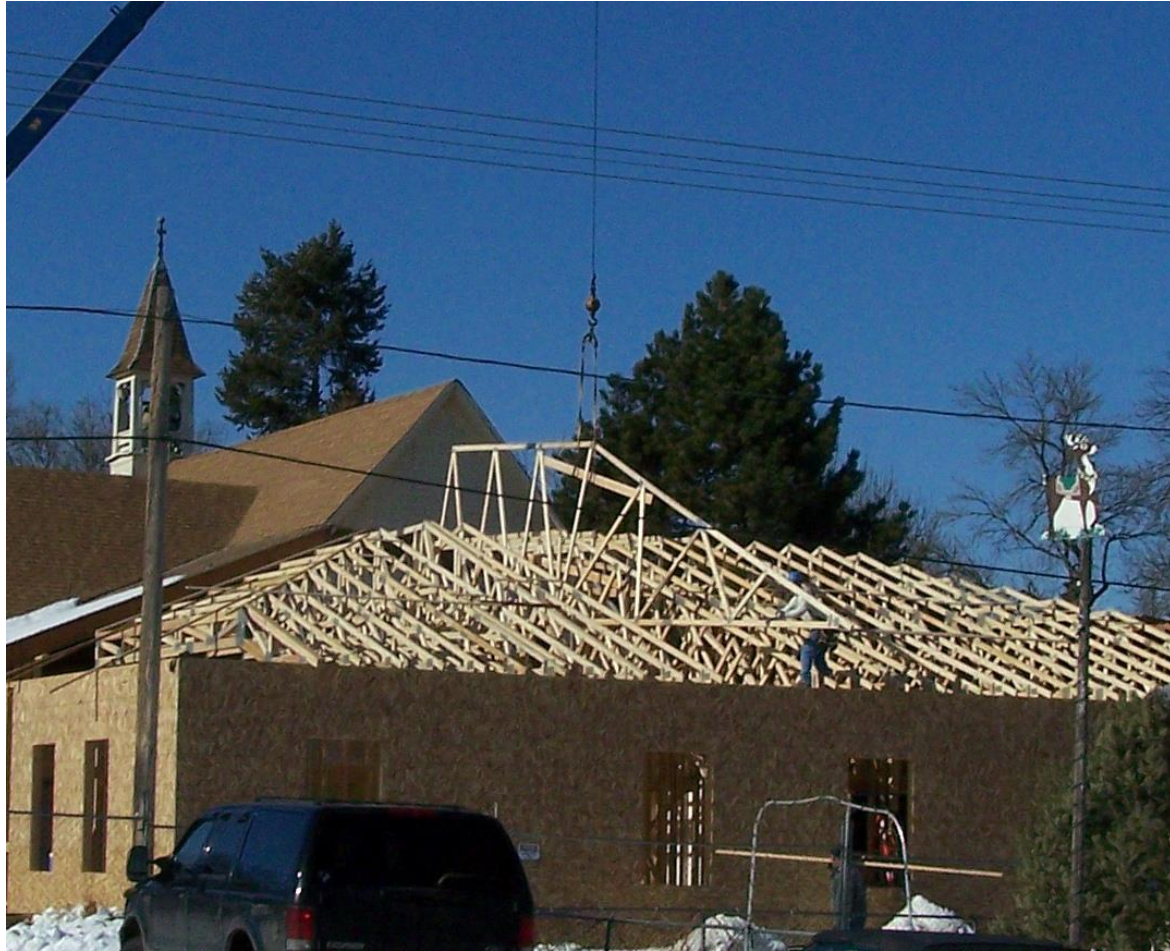
A roof truss being lowered into place by crane, over the Fellowship Hall.
