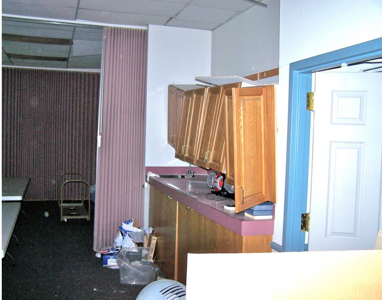
Fellowship Hall Damage GB – 102_1568
